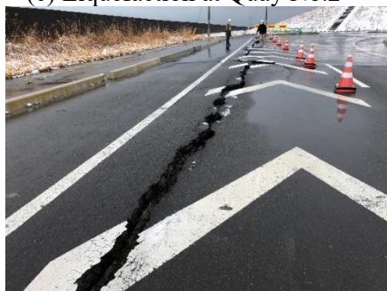
(e) Crack in the road at Quay No. 5
