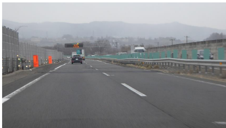
Figure 16. Road section near Box Culvert Kunimi 71, at 293.73 KP (37°59'39.5"N, 140°36'26.3"E): repaired crack
