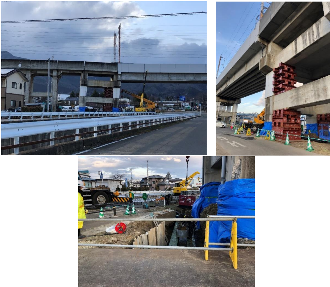
Figure 10. Damaged pier of the Tohoku Shinkansen viaduct
