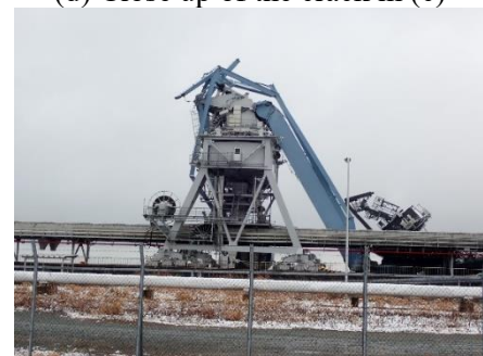
(f) Damaged coal unloading machine
