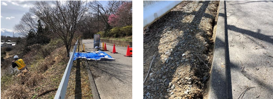
Figure 4. Ground settlement in Minamimachi
