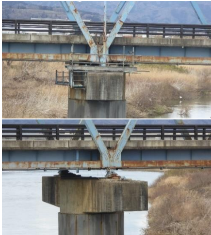
(c) Displacement in pier supports
