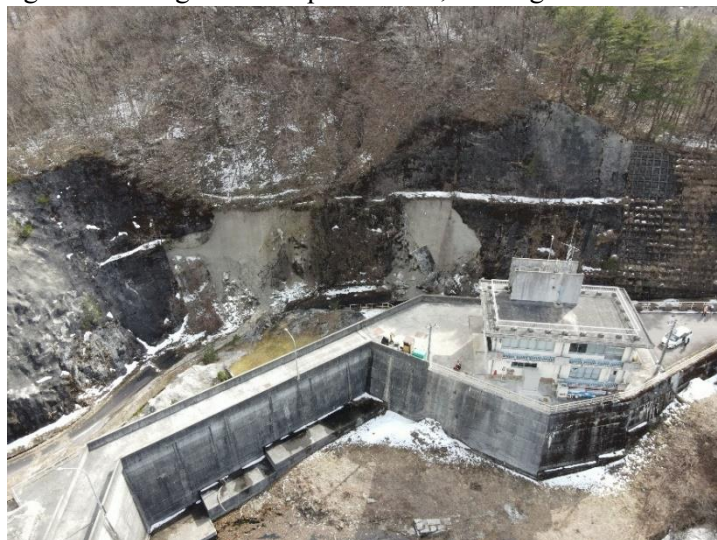
Figure 5. Landslide next to Dake Dam
