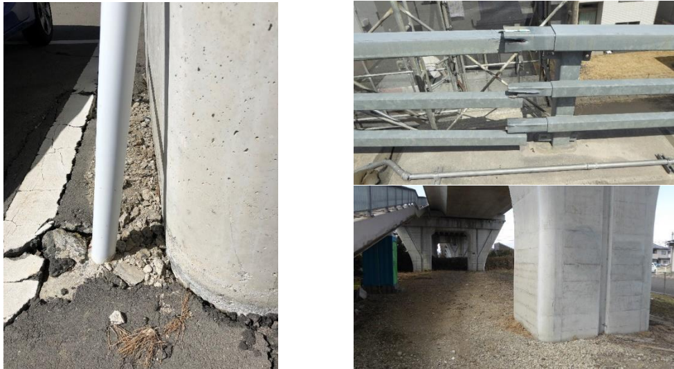
Figure 8. Damages in the Kasaishi Tohoku Line Overpass
