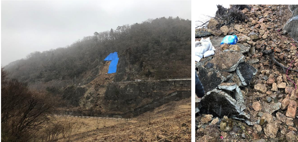
Figure 15. Landslide at Tarumizu Dam
