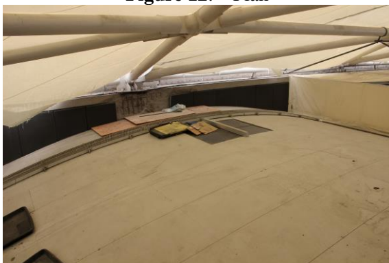
Figure 14. Damage to the bearing of the truss frame
