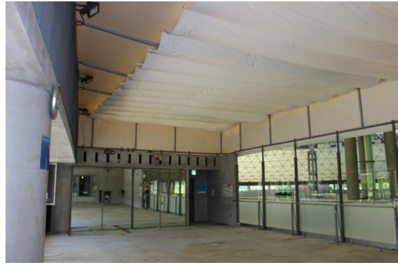
Figure 17. Damage to the movable membrane ceiling
