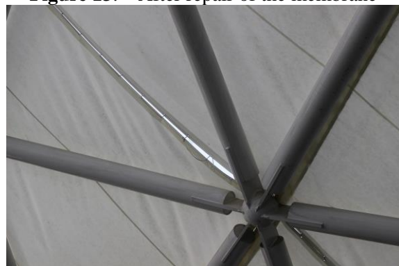
Figure 15. Frayed strings of the membrane
