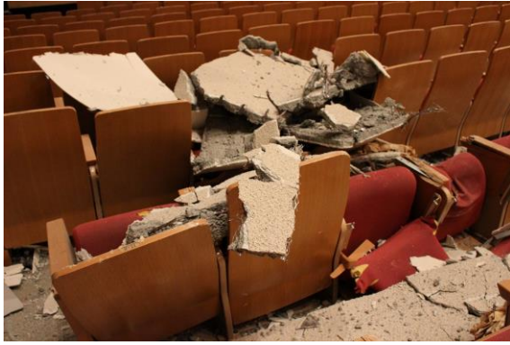
Figure 6. Damage to the audience seats
