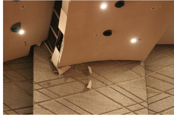
Figure 7. Failure of the ceiling
