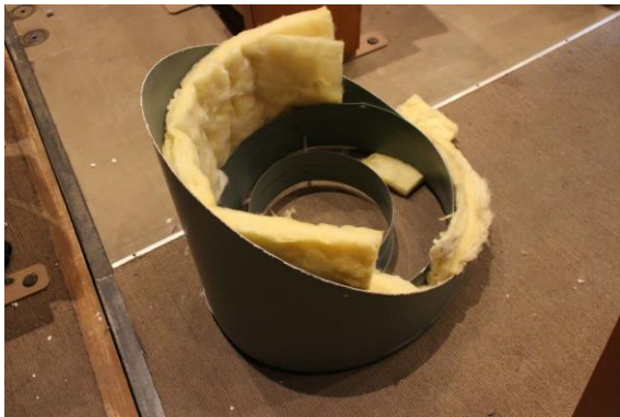
Figure 8. Fallen lighting cover
