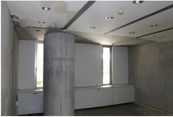
Figure 16. Damage to the ceiling
