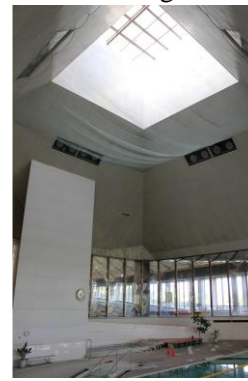
Figure 19. Safety net for ceiling collapse
