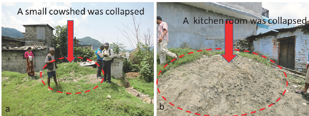
Figure 7 Typical effects of sinkhole on residential properties: (a) collapsed cowshed and (b) collapsed kitchen
