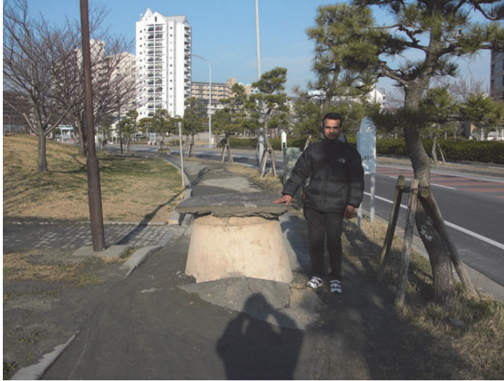
Figure 1 Manhole uplifted during the 2011 earthquake in Urayasu City
