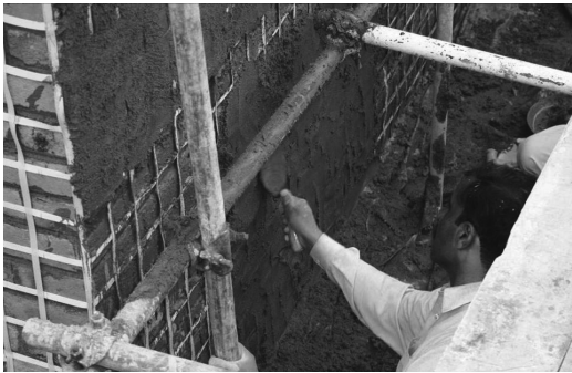
Figure 2. Field Application of PP-band retrofitting technique to a sample masonry house in Kashmir, 2005
