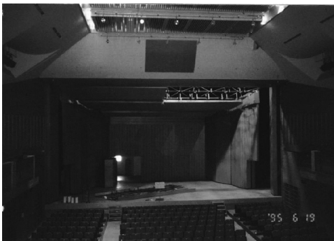
(a) Collapse of an acoustic panel
