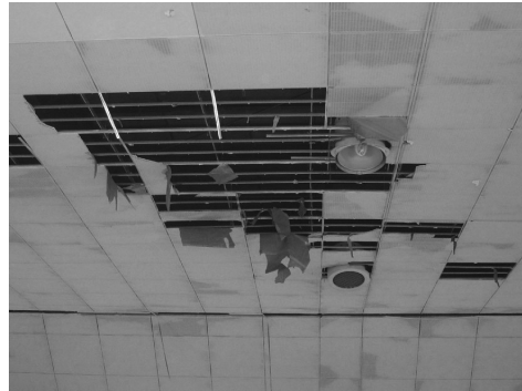
(b) Gypsum boards failed at the nails' heads
