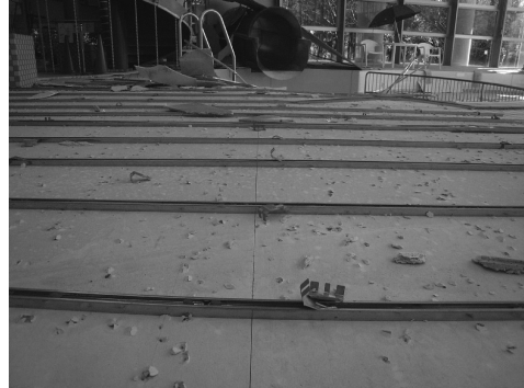
(b) Failed furring strips and clips
