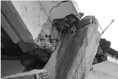
(a) Separation between beam and column
