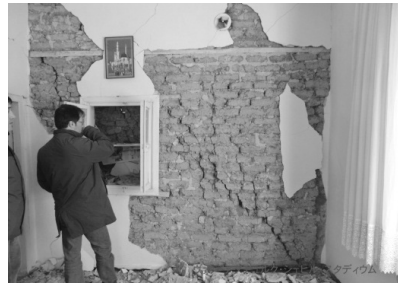
(b) Out of plane failure
