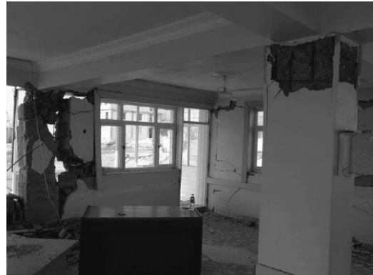
(b) Column flexural yielding at the top
