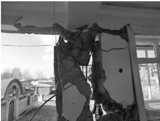
(a) West side column failing in shear
