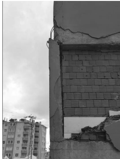
(b) beam-column joint failure (south-east corner of Building C)
