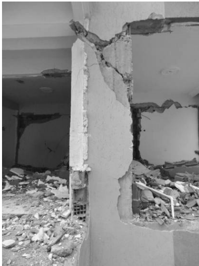
(a) shear failure of south side column of Building A (damage level V)
