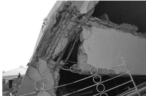
(b) Anchorage failure of beam main rebar
