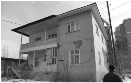
(a) Damage of adobe house
