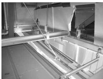
(c) Failure of the panels next to the smoke barrier
