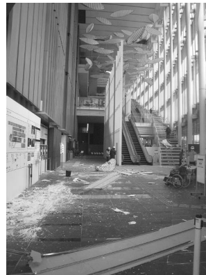
Figure 7. Internal view of the entrance hall after the disaster
