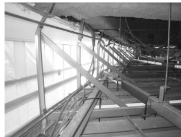
(d) Failure of the vertical panels in the vicinity of the facade
