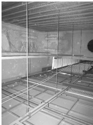
(a) Ceiling system
