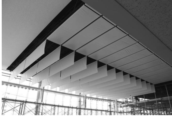
Figure 11. Recovery of the eastern ceiling at the entrance hall by membrane materials
