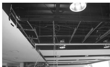
Figure 11. Deformation at northeastern corner
