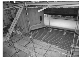
(c) Fallen curved surface ceiling
