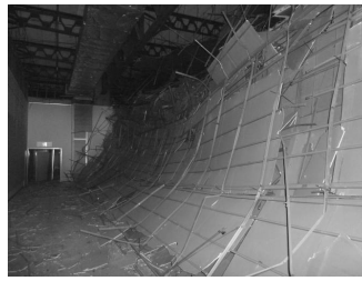
(b) Fallen ceiling
