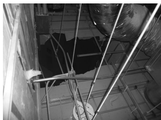
(c) Ceiling frame
