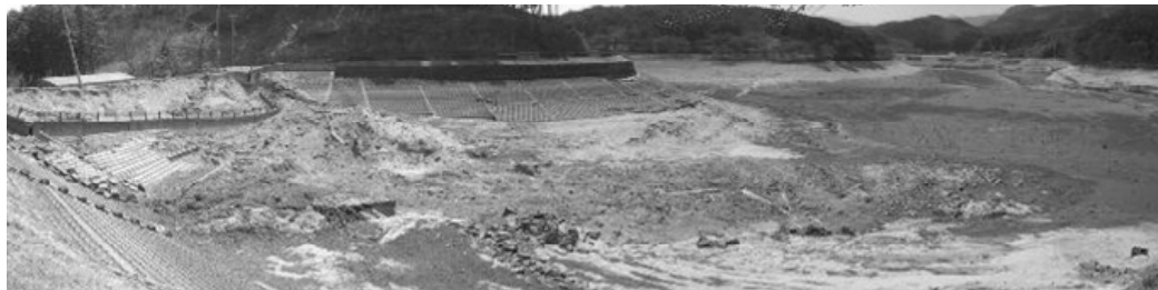
Photo 1 Upstream slope failure of the small dam (April 15 th at 37.299778, 140.195348)
