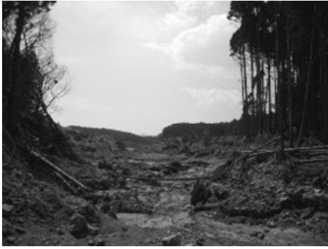
Photo 4 Breached dam body as seen from downstream (April 15 th at 37.302661, 140.196055)
