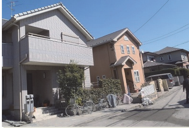
(a) Inclined and sunken houses Photo by Kiyota T., at 35.641895, 139.89886
