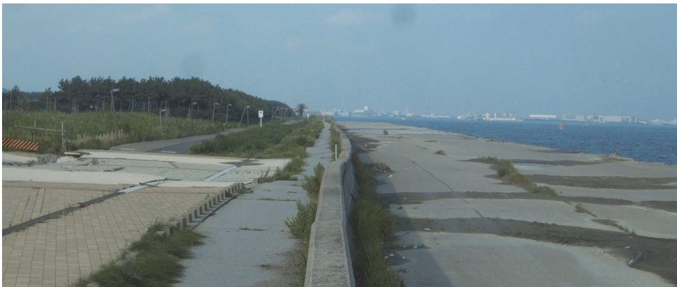
Fig. 7. Seawall pushed forward Photo by Konagai K. taken on Aug. 1 st , 2011 at 35.63666, 139.931638
