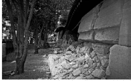
Photo 2. The rammed earth wall (“Oo-neri bei” in Nishinomiya shrine) collapsed by the Great Hanshin Earthquake Disaster. This photo was taken on January 17 1995 (by courtesy of Nishinomiya City)
