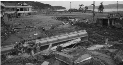
Damage to the Okirai elementary school. The students were safe even though the tsunami came.
