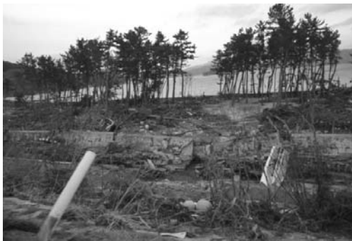
Damage to the tide embankment at Yamada bay
