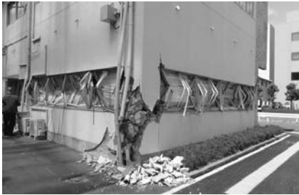
Damage to a 3-story reinforced concrete building due to ground motion
