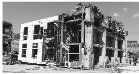
A four story steel frame building was overturned by the tsunami.
