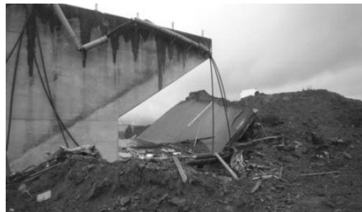
The tsunami destroyed the road bridge.
