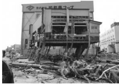
Fish processing facilities near the port were damaged.
