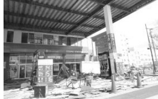
Collapsed ceiling at a gas station
