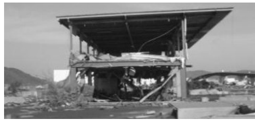
A damaged steel frame structure
