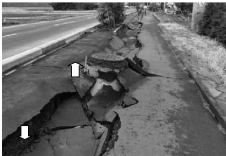
Photo 6. Uplift of sewer manhole and settlement of backfill soil in Naka city, Ibaraki prefecture (site TT)
