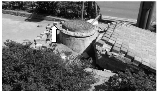
Photo 7. Uplift of sewer manhole in reclaimed land of Urayasu city, Chiba prefecture (site R2)
