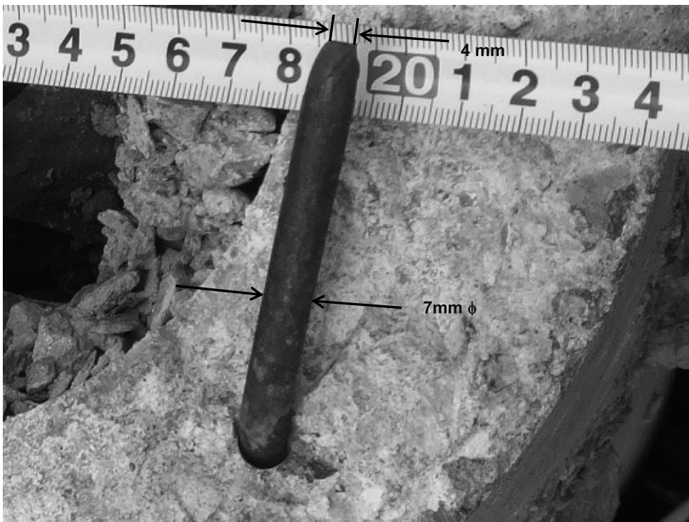
Figure 5 Fracture surface of PHC pile for Building #1: A fracture cross-section of PHC (Pretension type centrifugal High strength pre-stressed Concrete) pile used for Building #1, 300mm and 120mm in outer and inner diameters respectively, has 7 PC wires exposed with cut ends thinning to about 4mm diameter.
