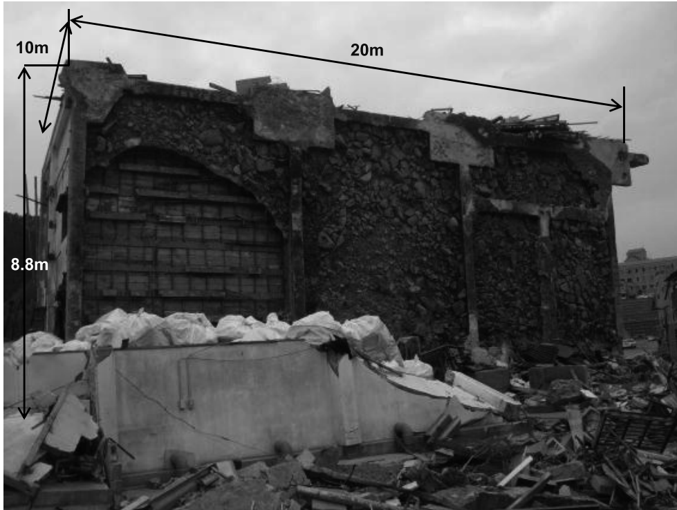
Fig. 9 Building #4: toppled west from its original Location at N38.440608, E141.446511. This was a steel-frame cold storage warehouse for fishes and seafood products. Dim marks of pile head are seen indicating the building was just resting on piles. This warehouse had a small door/window aperture.
