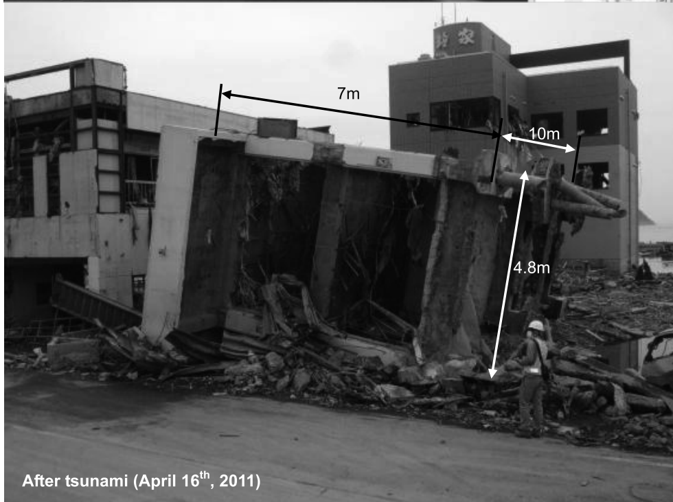
Figure 6 Toppled Building #2 (Onagawa Police Box, Original location at 38.445086,141.446760): Onagawa police box was overturned north. Piles were broken and upper halves of them were uprooted. There is a dent on the roof indicating that something massive was pushed against it.
