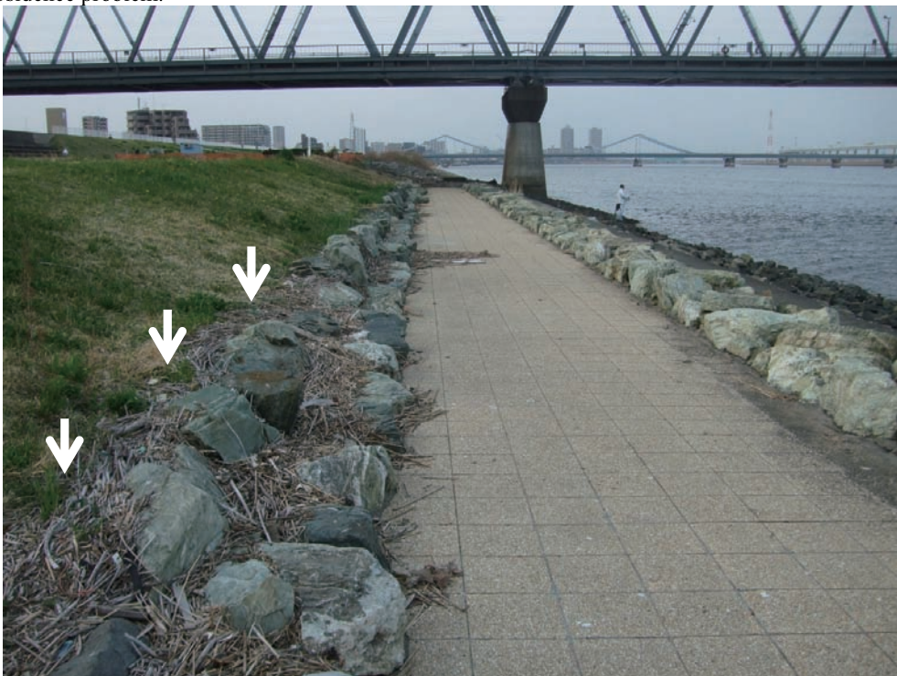
Figure 3(b) Tsunami marks along the right bank of Arakawa River
