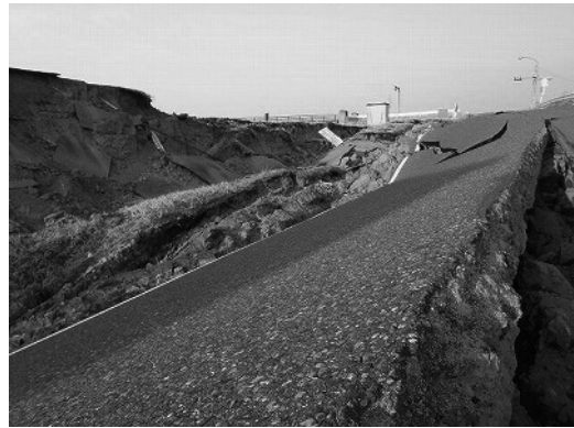
N38 31.810 E141 00.311 Photo 11 Damage to levee (Naruse River)
