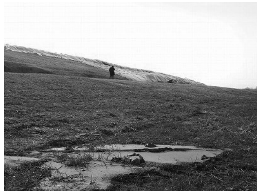
N38 31.705 E140 54.128 Photo 13 Liquefaction-induced damage of levee (Naruse River)
