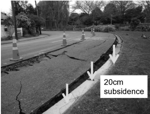
Photo 3 Road on river dike suffered from settlement and cracking (Site 63 in Fig. 4)
