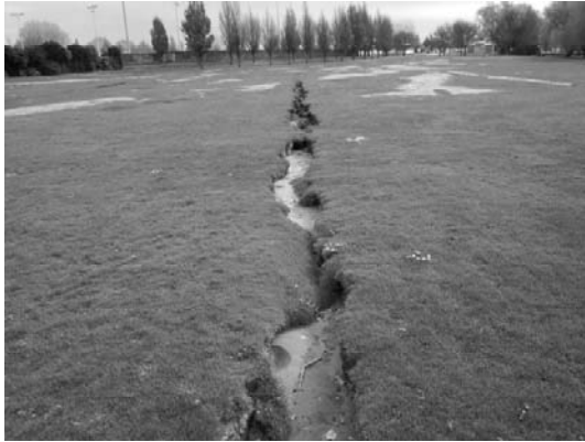
Photo 10 Number of cracking and boiled sand could be observed in Porritt Park (Site 20 in Fig. 6)
