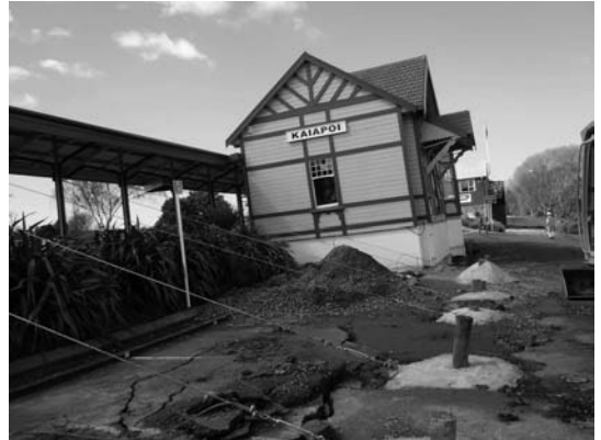
Photo 13 Boathouse suffered uneven settlement due to liquefaction (Site 109 in Fig. 15)
