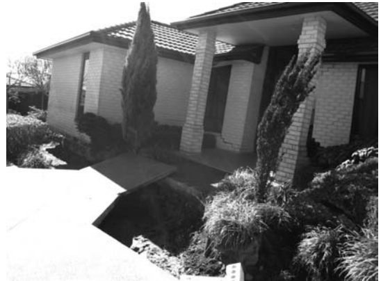
Photo 15 Damaged house due to liquefaction-induced ground deformation (Site 117 in Fig. 15)
