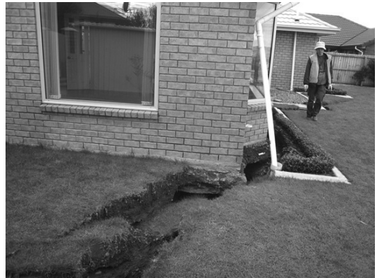
Photo 12 Foundation of house suffered from large cracking (Site 93 in Fig. 11)
