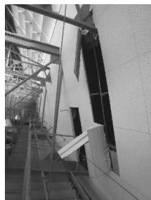
(e) Failure of vertical panels in roof space
