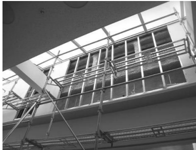
Figure 12. Public Complex – Failure of facing panels in the joint of two buildings on the 2nd story
