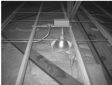
(c) Lighting equipment under the roof
