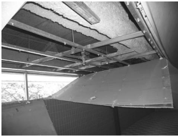
(a) Failure of panels
