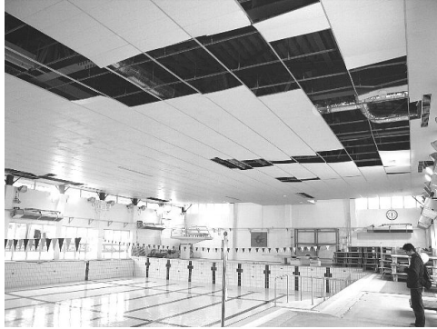
Figure 13. Example of damage to line-type ceiling (The Niigataken Chuetsu-Oki Earthquake in 2007)
