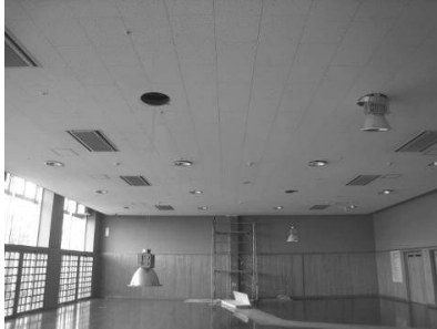
(a) Failure of lighting equipment and ceiling panels around a steel column
