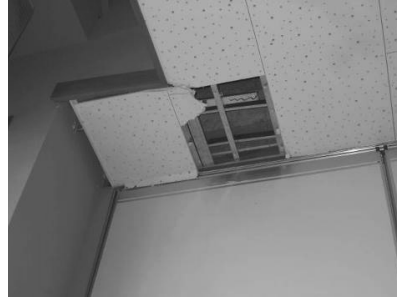
(b) Failure of sliding walls and a ceiling panel
