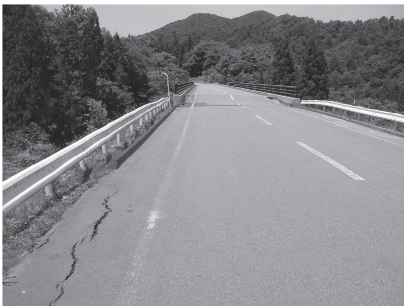
Photo 5. Settlement of approach embankment for Tochinoki bridge along national highway route No. 398 (site B in Figure 2)
