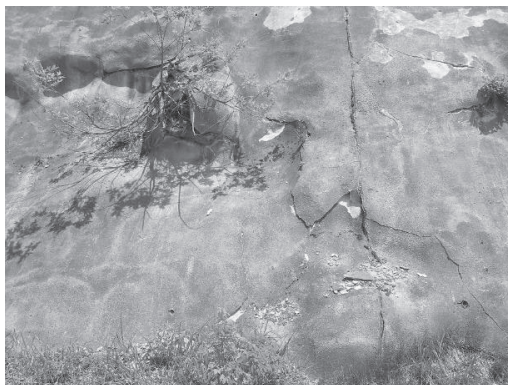
Photo 10. Cracks in shotcrete on cut slope
