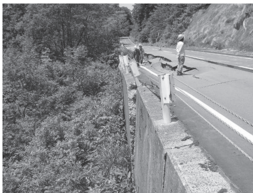
Photo 9. Tilting and settlement of gravity type retaining wall in Photo 8
