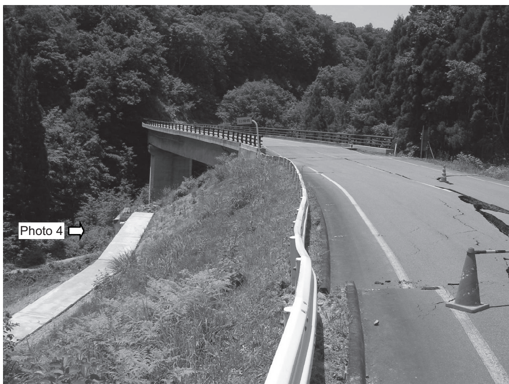
Photo 3. Settlement of approach embankment for Shirakaba bridge along national highway route No. 398 (site B in Figure 2)
