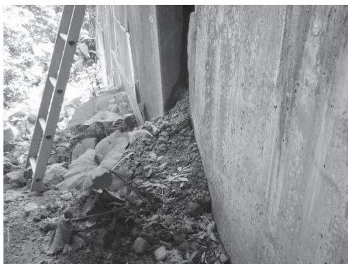
Photo 7. Outflow of backfill soil between reinforcement frame and original wing of Tochinoki bridge
