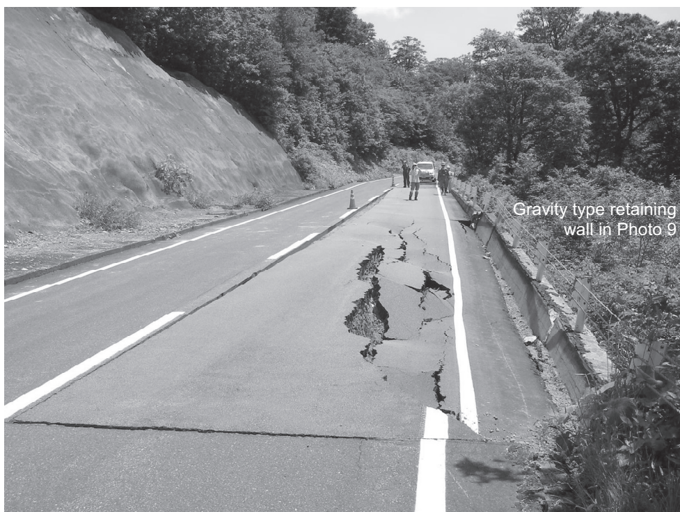
Photo 8. Collapse of embankment along national highway route No. 398 (site C in Figure 2)
