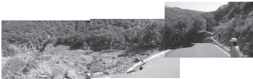
Photo 11. Large slope failure including embankment along National Highway route No. 342 (site D in Figure 2)
