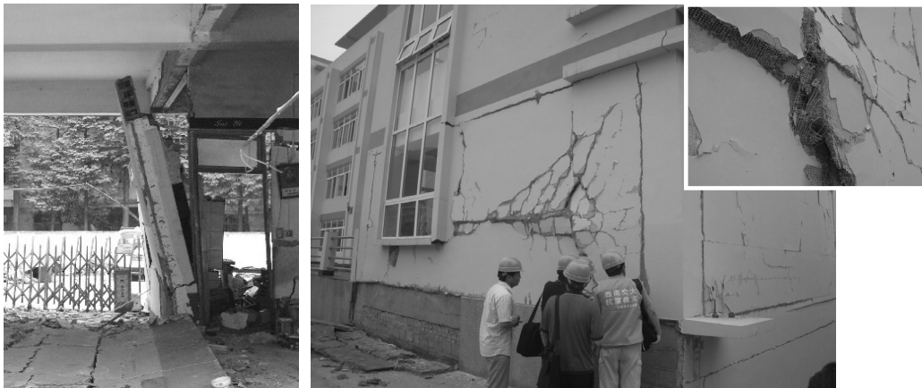
Photo 3 Failed brick wall (left) and survived brick wall (right)
