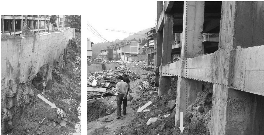
Photo 9. Structural damage due to failure in retaining wall
