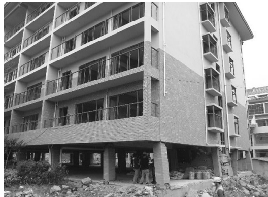
Photo 6. Soft first story of a 6 story RC apartment house
