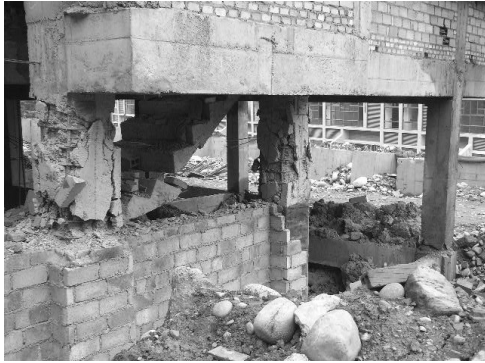
Photo 4. Typical shear failure in RC short columns
