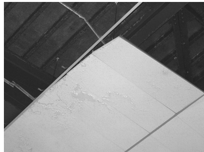
(b) Collapse of ceilings 2
