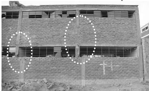
Figure 18. Bad construction example in Los Molinos, Ica
