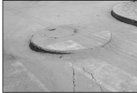
Figure 9. Manhole pushed up and surrounded by ejected fine sand, northwest of Pisco
