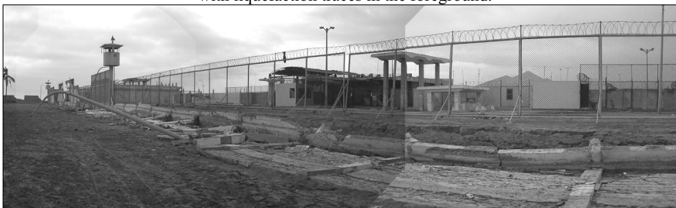
Figure 7. Collapsed wall at Chinchá Prison due to large ground deformation
