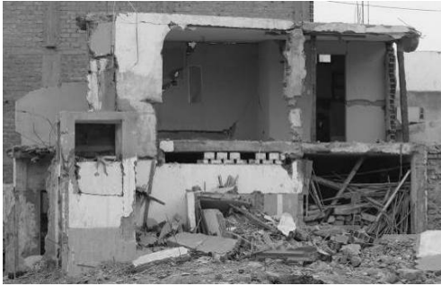
Figure 14. Load bearing wall made of pandereta bricks and poor steel reinforcement in the confinement (Pisco, Ica)
