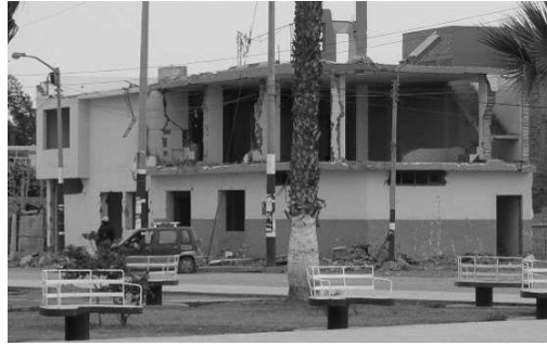
Figure 15. Collapsed façade wall due to lack of confinement (Sunampe, Chincha)
