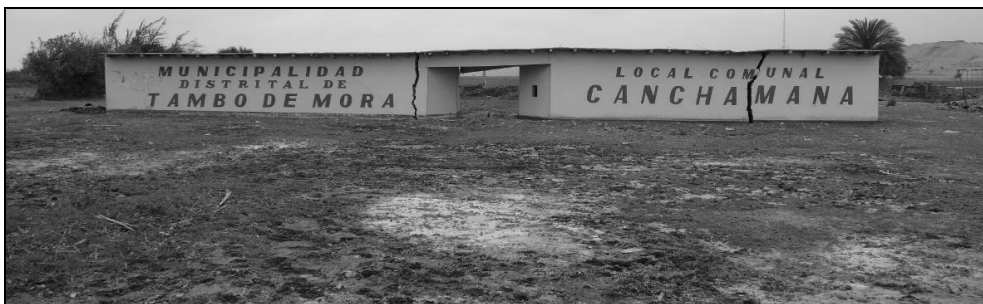
Figure 6. Severely damaged community building in Canchamana, with liquefaction traces in the foreground.
