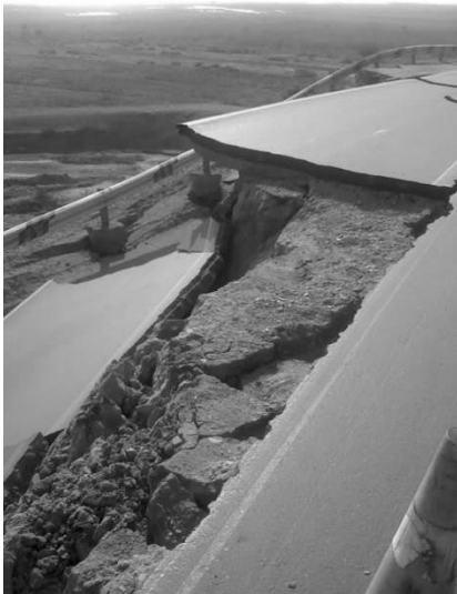
Figure 20. Slope failure caused by liquefaction induced lateral spreading
