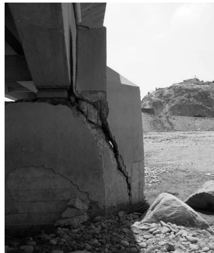
Figure 24. Failed wing with poor reinforcement (pillar with movable bearing)
