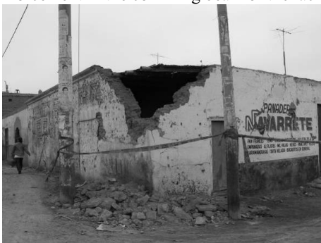
Figure 12. Corner collapse in adobe house (San Luis, Canete)
