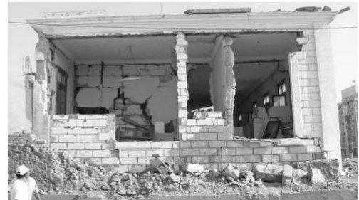
Figure 17. Concrete block wall collapsed out-of-plane (San Juan de Dios Hospital)
