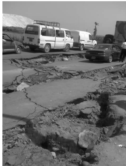
Figure 21. Liquefaction induced embankment failure
