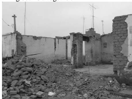
Figure 13. Collapsed adobe house (Nuevo Monterrico, Canete)
