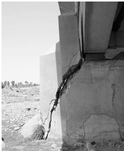
Figure 23. Failed wing with poor reinforcement (pillar with movable bearing)
