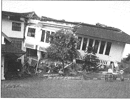
Photo 31. A damaged government building at Site W
