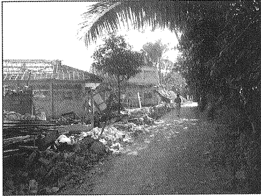
Photo 13. Damaged primary school at Site I
