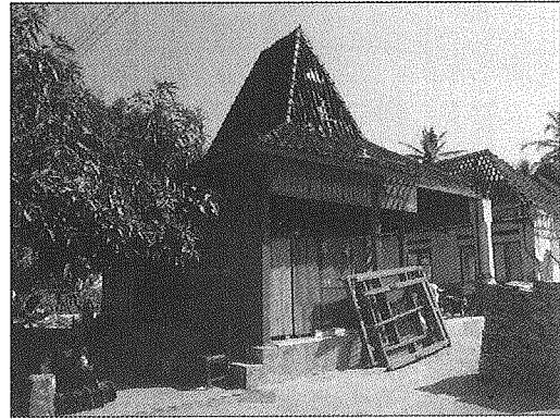
Photo 28. A damaged traditional house at Site T
