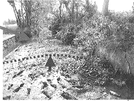
(b) Bottom of stream along the road has been pushed up
