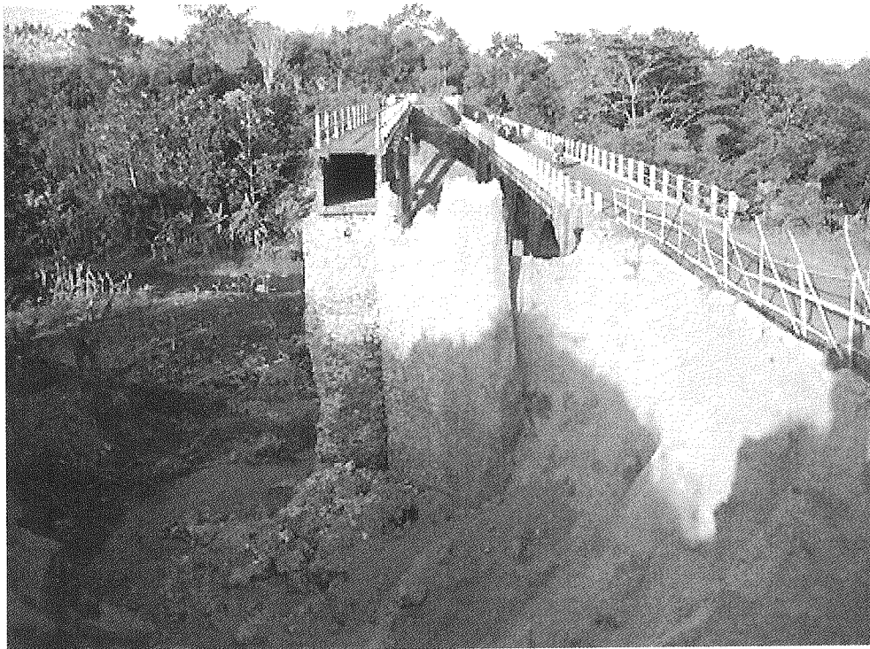
Fig. 4. Mataram canal bridge: Soil mass of right embankment behind masonry abutment has gone.
