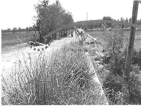
(a) Location of skewed bridge: Edge lines of road are seemingly dislocated right-lateral. However no clear dislocation was found in rice paddies.
