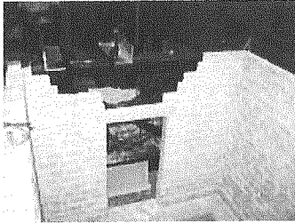
Photo 1: Partial Collapse of Non-retrofitted Building Model at the 44th run (Seismic Intensity, 4 JMA Scale)
