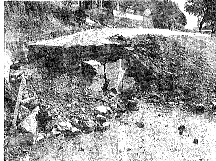
Fig. 33: Road No. 6, north of Balakot (Site B in Fig. 36)
