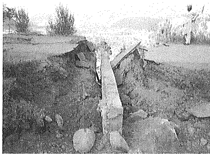
Fig. 22: Collapse of a culvert on a local road in south of Balakot
