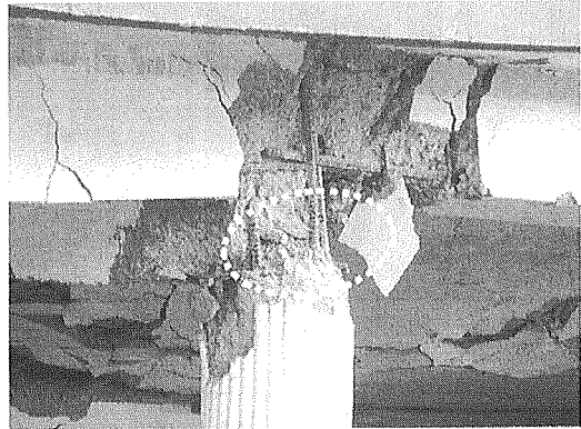
Photo 11-2. Beam rebar terminated at column surface
