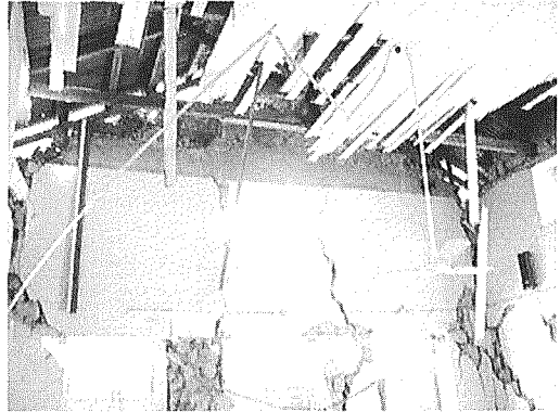
Photo 8-4. Damage to URM wall
