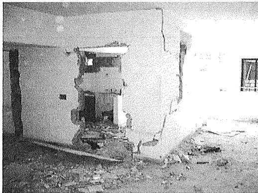
Photo 1-2. Damage to URM walls
