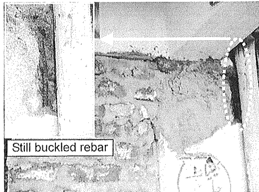
Photo 10-6. Inadequate repair at column top
