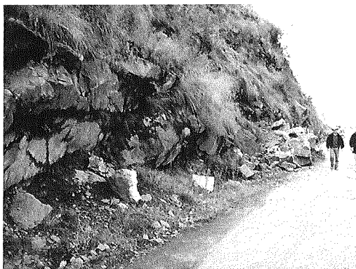
Fig. 15. Blocky rock mass along western mountain side of Jehlum valley: Water is seeping through cracks
