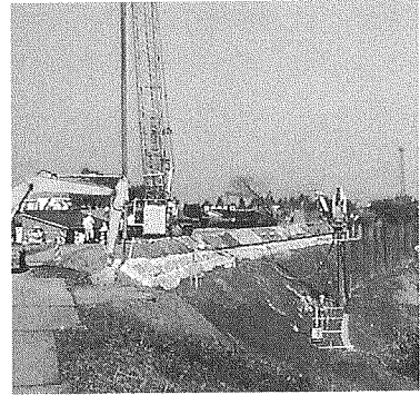
Figure 18. Rehabilitation work of a dike along the Kariyata river (at Gohyaku-kari, Nakanosima-machi; site 11 in Figure 1)
