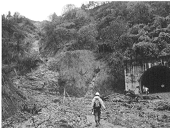
(a) Debris flow bed exposed by the tunnel mouth
