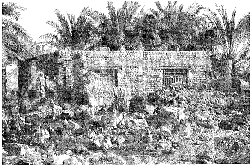
Figure 11. Completely collapsed adobe house
