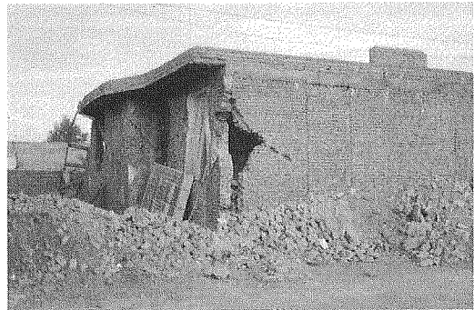
Figure 12. Heavily damaged partially confined masonry house
