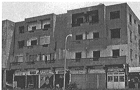
(a) Structure 1 (4-story RC structure with soft floor type of damage)
