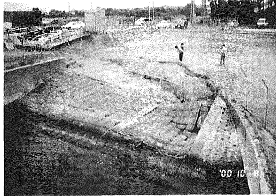
Fig. 11 Lateral flow at Nakaura water gate
