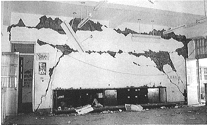
Damage Class IV
