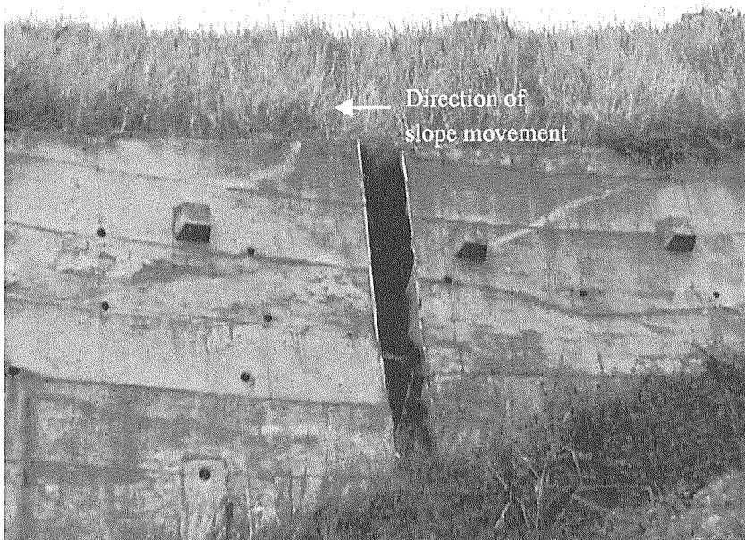
Plate 2. Opening at construction joint of anchored RC retaining wall due to large-scale slope movement (at an embankment along District Road No. 129; site 2 in Fig. 1)
