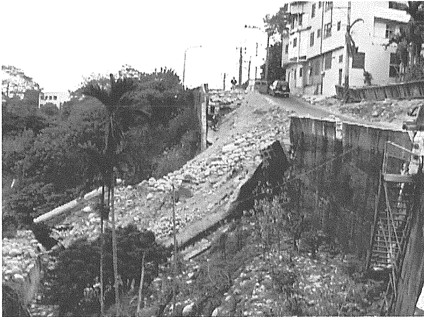
Plate 1. Collapse of RC retaining wall due to permanent ground displacement along fault (along a road on the south of Chang-Geng Bridge; site 1 in Fig. 1)
