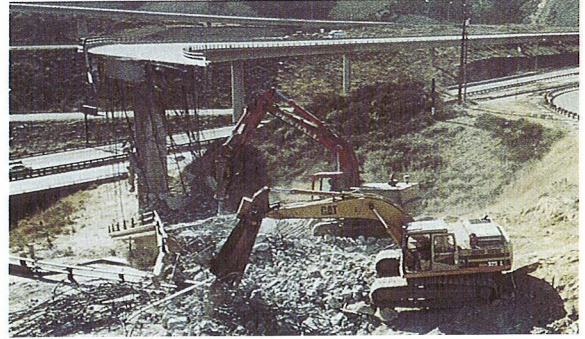
Northridge earthquake, 1994 (USA)
