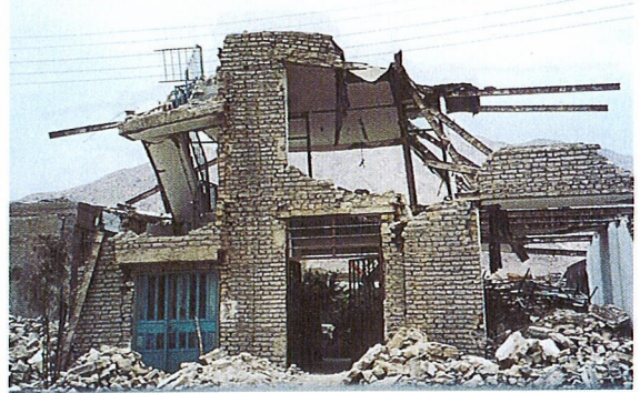
Qayen earthquake, 1997 (Iran)
