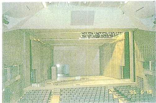
fig.3 Fallen acoustic boards
