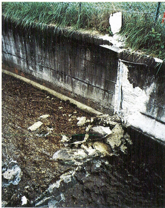
Photo 2 Damaged concrete wall of drain
