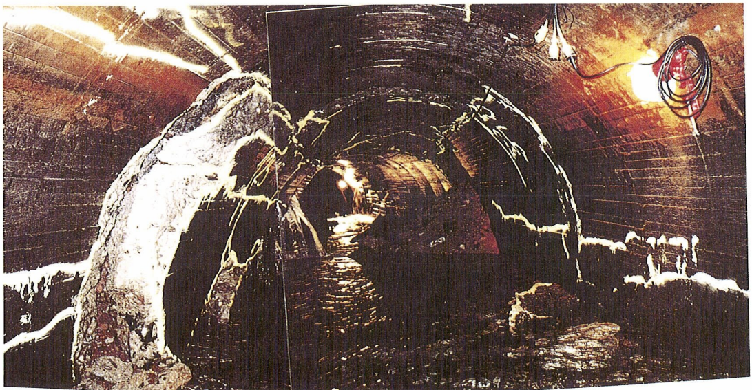
Photo 4 Damage to outlet tunnel (provided by Tohoku Electric Power Company)
