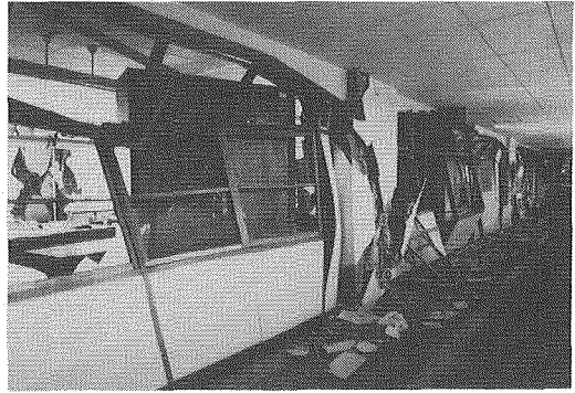
Photo. 2 Interior view of collapsed Hachinohe-higashi High School. (Photo by Daily Tohoku)
