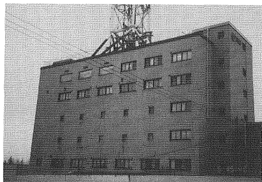
Photo. 12 Shear cracks in columns and walls. Building No. 3 of the NTT Hachinohe Office
