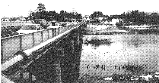
Photo.23 Sunk and tilted pier 3 of the Ohashi bridge
