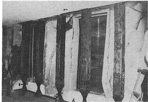
Photo. 10 Temporary retrofit with steel columns to support the second floor in Hachinohe Commercial and Industrial Association Office. (Photo by Kazuhiro Kitayama, Tokyo Metropolitan University)
