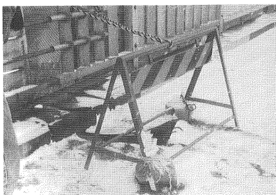
Photo.25 Damage to the steel deck plate of the Hachinohe-Ohashi bridge
