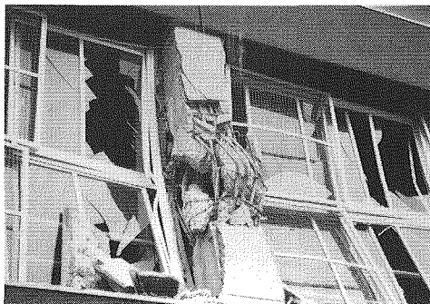
Photo 11: Failure of a column of the gym.
