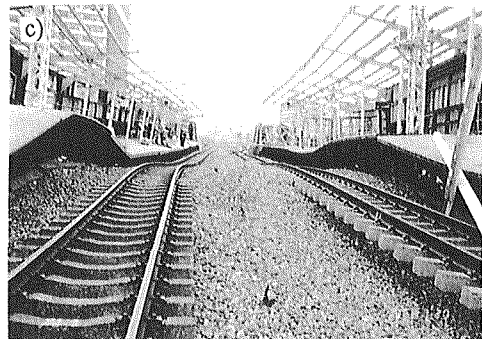
Fig. 10 Rupture of the facing of cantilever RC RW; embankment of JR Shin-Nagata Station (Site CL2 in Fig. 2); a) sketch and b) picture of damaged RC RW, and c) view of the previous Shin-Nagata station
