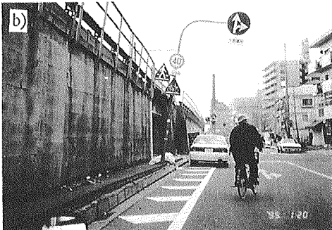
Fig. 9 Typical damage to cantilever RC RWs for embankment of JR Sanyo Line between Hyogo and Shin-Nagata Stations (Site CL1 in Fig. 2); a) sketch and b) pictures
