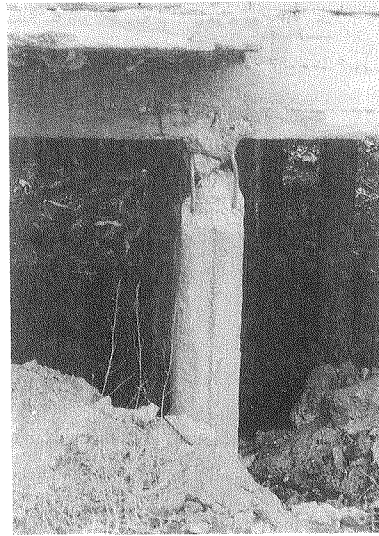
Photo 7: Shear failure at the top of column
