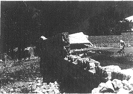
Photo 23 Blocked stone boundary wall, Arandu
