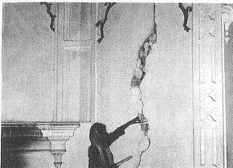
Photo 9 Damage to engineered structure
