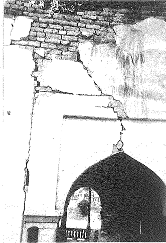
Photo 12 Arch failure, Old Fort, Chitral
