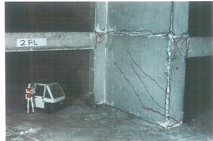
Photo. 4 Cracks at the First Story (the SHIFTED) (Plastic models are 1/20 scales)
