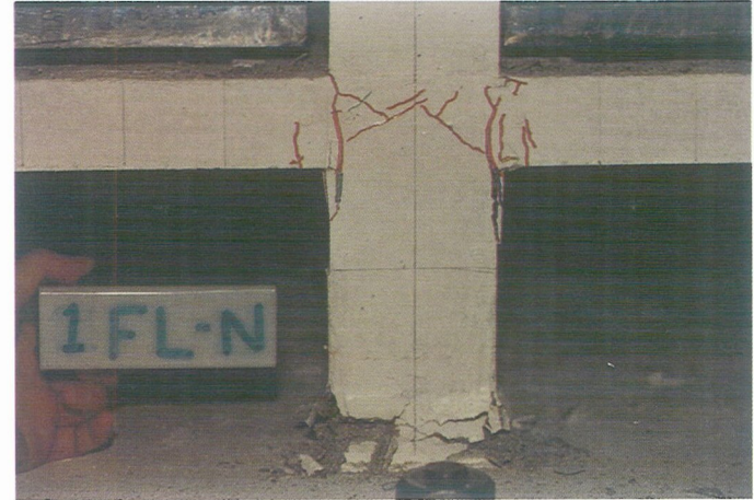
Photo. 3 Cracks at the Bottom (the STANDARD)
