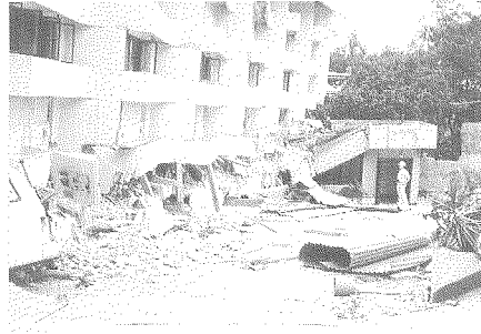
Photo 40 Collapse for first two stories of Nevada Hotel building
