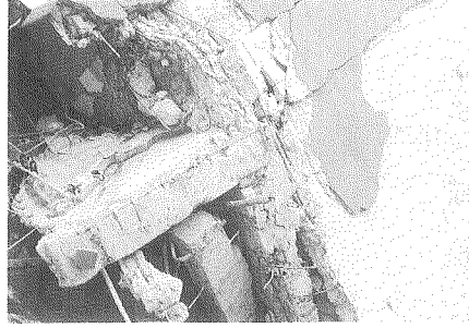
Photo 27 Damaged beam column joint showing beam reinforcement extensions not confined in column cage
