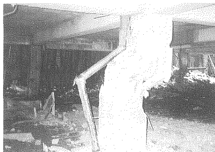
Photo 22 Severe shear failure of columns at the basement of S & L building
