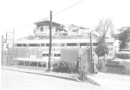
Photo 39 This Nevada Hotel building tilted and the penthouse damaged
