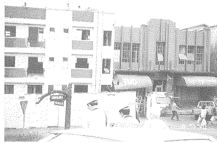
Photo 47 Plastic hinge formation of first floor column of Cafe Amapola (building on left is Siesta Inn)
