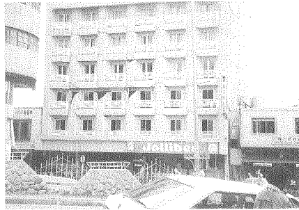
Photo 25 The Jollibee building across the Skyworld building suffered only damage to non-structural walls
