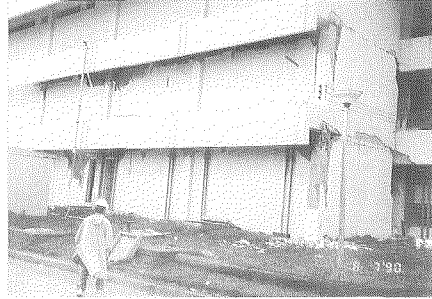
Photo 33 Damage to EPZA North building
