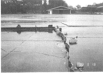
Photo 52 Extensive crack in runway of Baguio (Loakan) Airport
