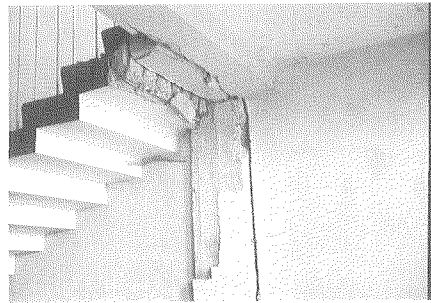
Photo 20 Crushing of concrete at stairs support of Little Angel's Nursery School
