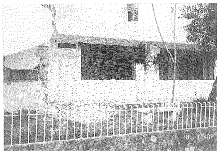
Photo 43 Shear damage to walls and columns in Quezon Hall at Teacher's Camp
