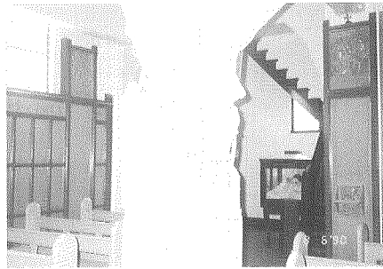
Photo 18 Shear failure of column supporting balcony at Baguio Cathedral
