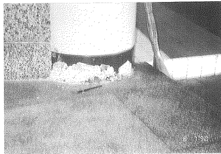
Photo 31 Void at bottom of column in St. Louis University (Boys' Campus)
