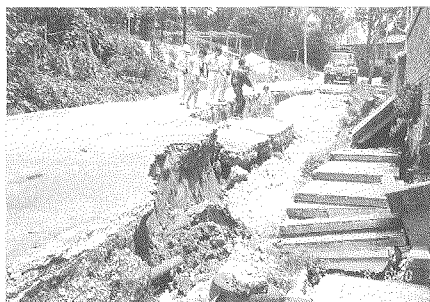
Photo 21 Ground subsidence of 1 to 3 meters can be observed around the S & L building front entrance
