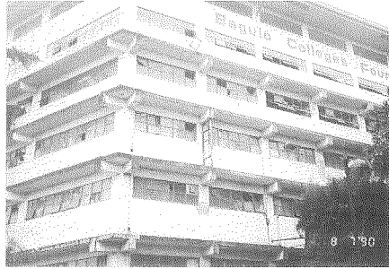
Photo 51 Slightly damaged building of Baguio Colleges Foundation next to collapsed building
