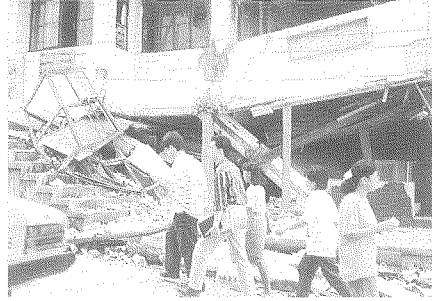
Photo 6 Side view of FRB Hotel showing the displacement of a circular column
