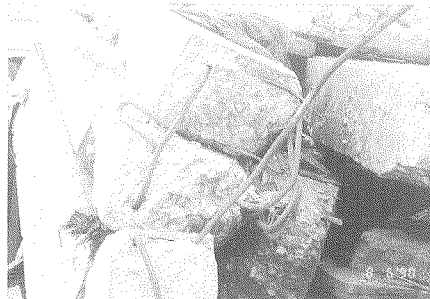
Photo 16 RC columns from Aurora Theater showing reinforcements and concrete with light brown color
