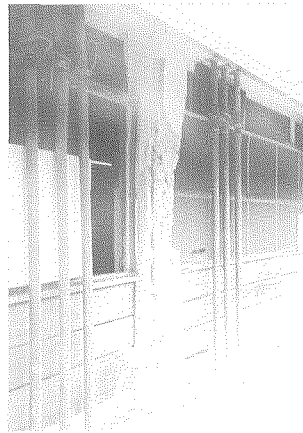
Photo 34 Exposed reinforcements of column in EPZA North building
