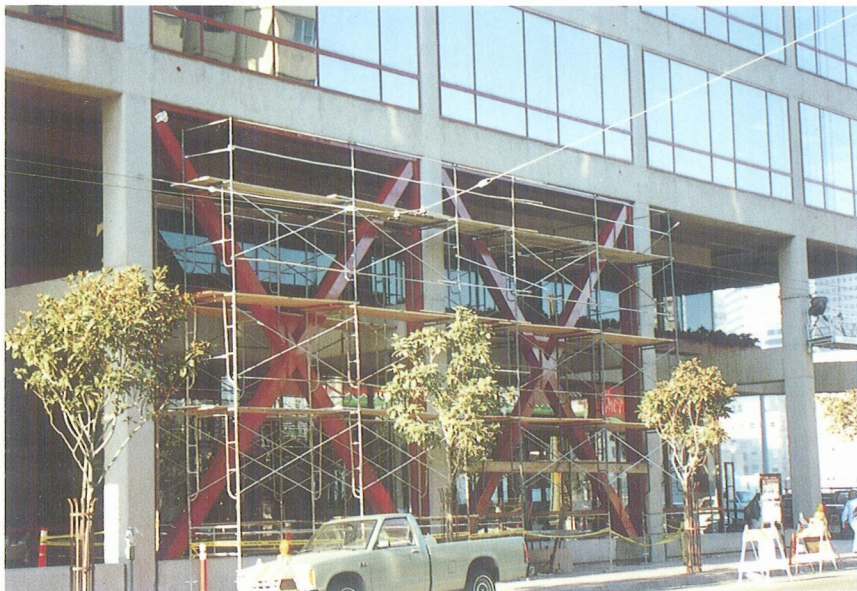
Photo 10. This relatively new reinforced concrete building at 4th and Harrison Streets in San Francisco had been strengthened and stiffened using steel brace systems before the earthquake. A large local buckle, however, developed in one of the brace systems and it was replaced immediately after the earthquake.
