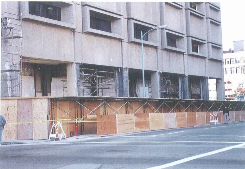
Photo 12. A steel frame building at Franklin Street and 17th Street in Oakland constructed in the early 1960s suffered major shear cracks in the lightweight concrete walls and columns. The damaged elements were under repairing when the investigation team arrived at the site.
