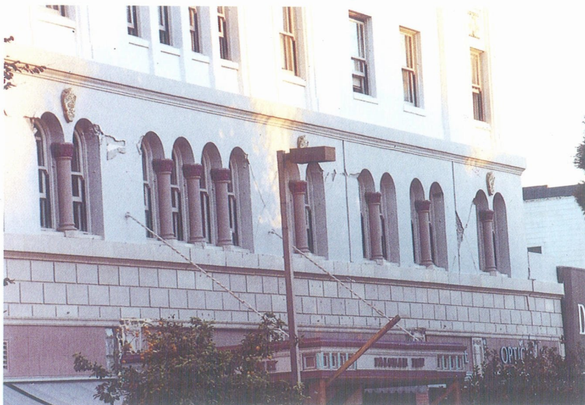
Photo 16. Old buildings on the Pacific Garden Mall in Santa Cruz suffered most severe damages in the epicentral region. This seven story old reinforced concrete hotel (Palomar Inn) suffered crackings in all of the shear walls at the second story. A few people were killed in this area.
