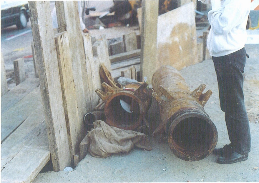
Photo 7. San Francisco's auxiliary water line broke at the south of Market Street. Due to the break of 12 inch high pressure line, water pressure of the fire fighting system dropped. Thus a fire boat was brought in for the fire fighting in Marina District.
