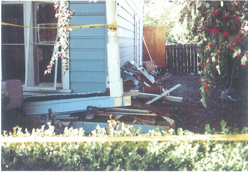
Photo 15. Another typical damage in the epicentral region was found in old wooden frame residential structures built on the cripple (or pony) walls of approximately 50cm high. These walls had poor lateral resistance and collapsed during the strong shaking.
