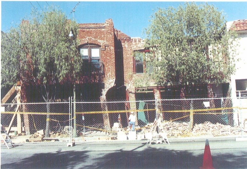
Photo 14. Unreinforced masonry buildings in the epicentral region suffered severe damages and partial collapses such as out-of-plane failure in parapets and the upper portion of the wall. This building on the main street in Los Gatos was extremely deformed in the first story.
