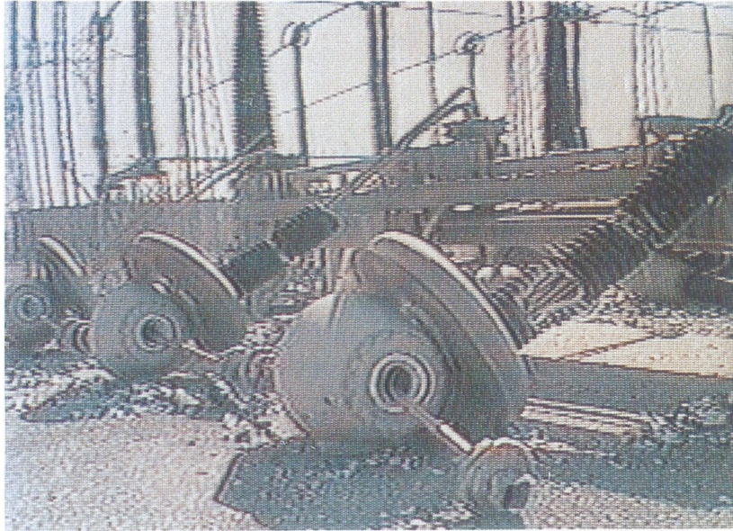
Photo 5. Three major substations, Metcalf, San Mateo and Moss Landing, were severely damaged in their switchyards, then about 1.4 million customers lost electric power. Top heavy circuit breakers turned over and oil leaked from transformers. (From the video tape of PG&E)
