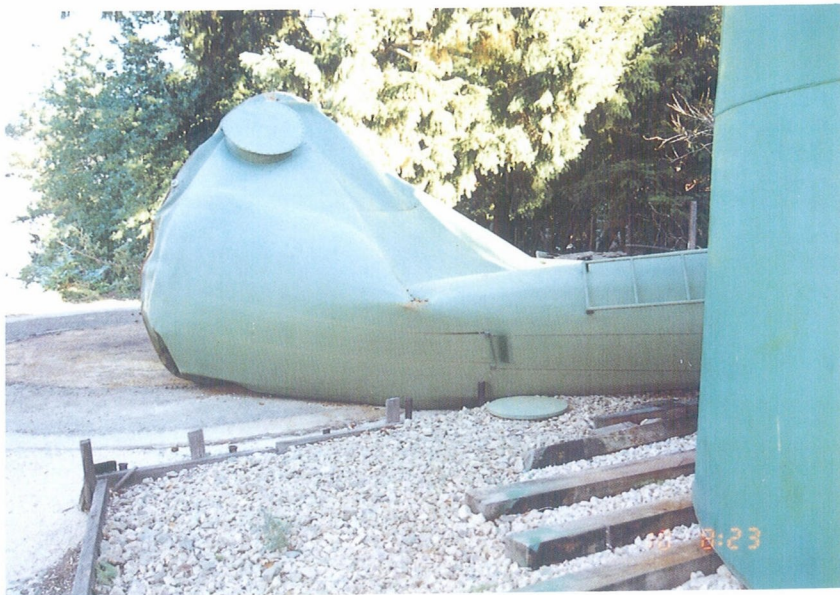
Photo 2. Water tanks by the Summit road running along the San Andreas Fault were severely ruptured. The 20,000 gallon water tank was shifted in the direction of N75^{\circ} E about 120cm on the timbers. The bottom plate of the 18,000 gallon water tank in the background was peeled off from the concrete foundation.
