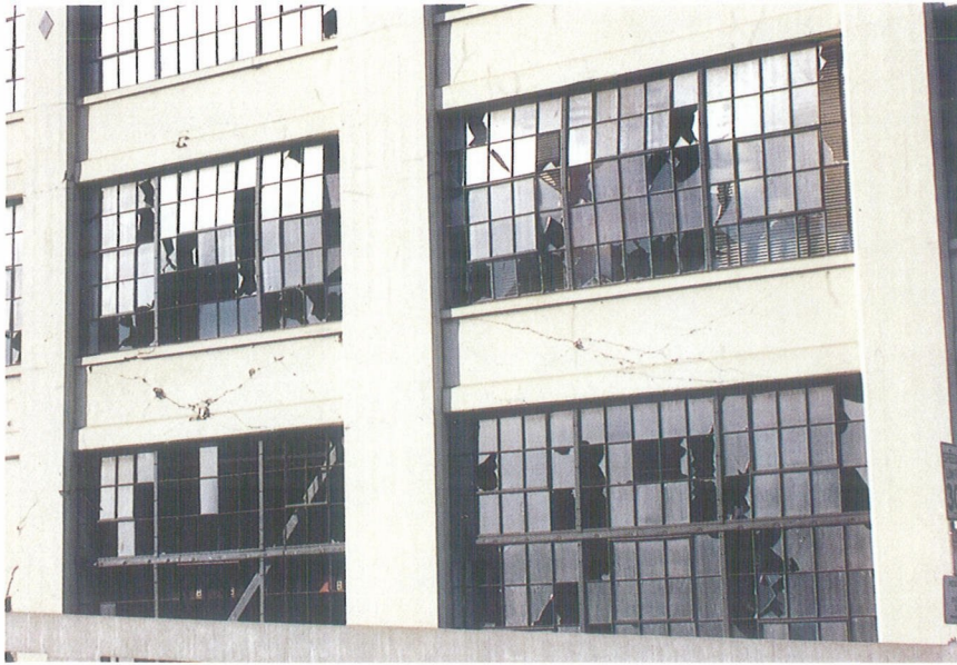
Photo 13. An old reinforced concrete warehouse in Emeryville suffered severe shear cracks in beams, columns, and walls. A highrise building, which is several hundred meters away from this building, experienced a strong ground motion, with a peak acceleration of 0.22g at the ground floor.
