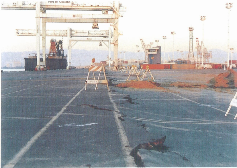
Photo 3. The backfill of the container pier in the Port of Oakland was settled about 1 to 1.5 feet resulting in cracks of piles supporting this pier and a tilt of cranes with their sea-side wheels on the pier and inshore-side wheels on the backfill.
