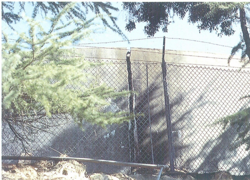
Photo 6. A prestressed concrete water tank broke from top to bottom and the full storage water flew out in Los Altos Hills. This tank of 1 mega-gallon was located unfortunately just above an extended fissure.
