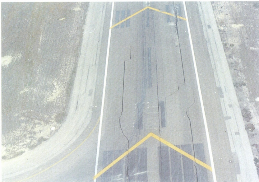
Photo 8. In Oakland International Airport, 3,000 feet of the 10,000 feet main runway were severely damaged. An extensive cracking was developed and many sand boils were observed. However, the airport was kept open except for very large aircraft.
