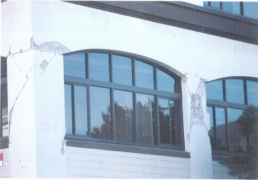
Photo 11. Shear cracks developed in the second story of a relatively new reinforced concrete building at Oak Street and Gough Street in San Francisco, mainly due to the presence of shear walls in the first story.
