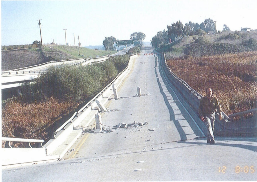
Photo 1. The slab of the Narrow Bridge of California State Highway 1 fell onto a wet low ground in Watsonville where many wooden and masonry buildings in the downtown area were severely damaged. The slab was punched by RC piles with diameter of about 37cm.
