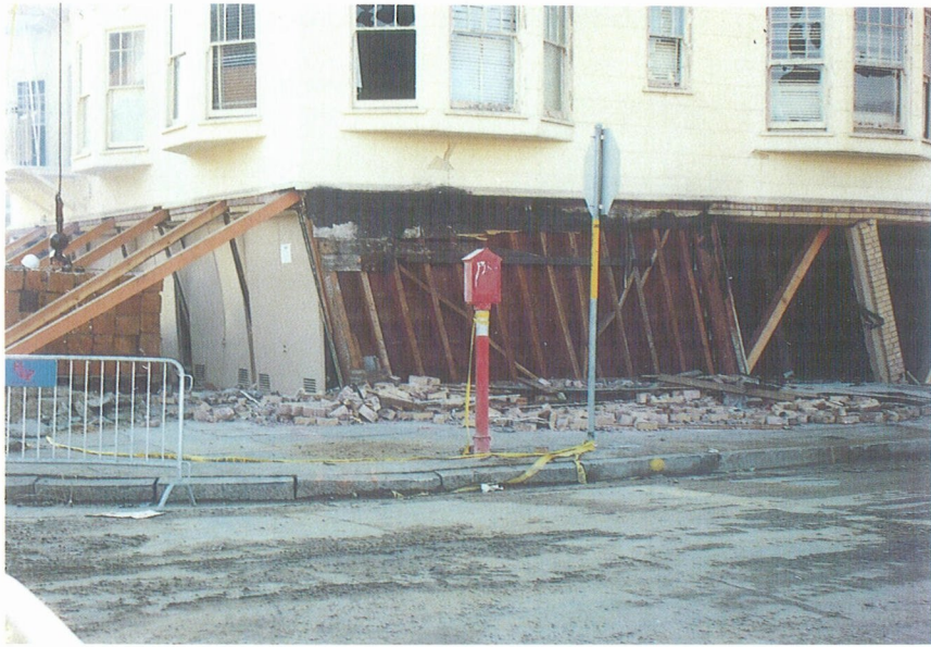
Photo 9. In Marina District, corner buildings were severely damaged. Most of them were 3 or 4 story apartment buildings in which the first story was taken up almost entirely by garages. The ground story had less lateral resistance than the upper stories and thus resulted in the "soft first story" behavior.
