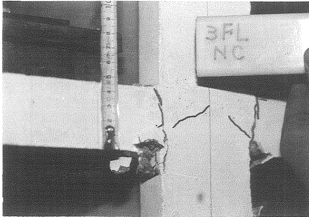
Photo. 4 Cracks at Beam Ends
