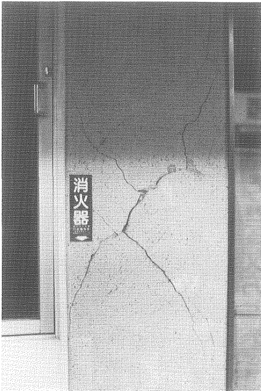
Photo. 4 X-shaped shear crack on a column in Chonan town hall
