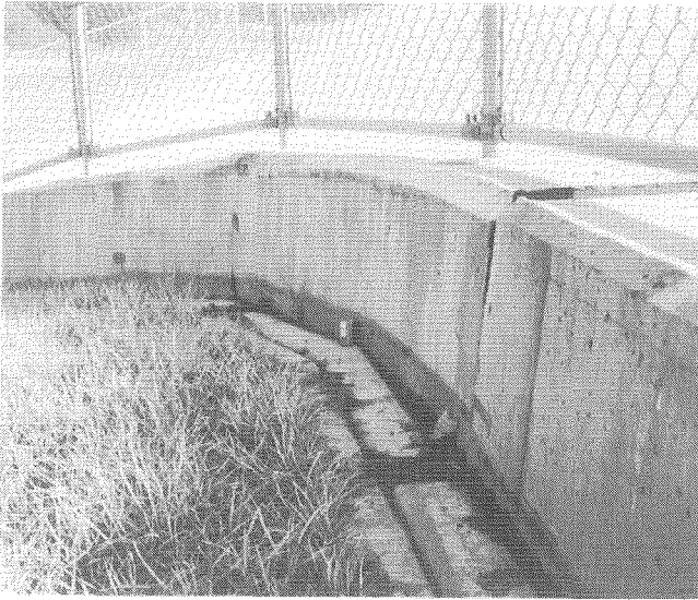
Photo. 10 Backfill of spillway(subsided to an extent of about 10cm)
