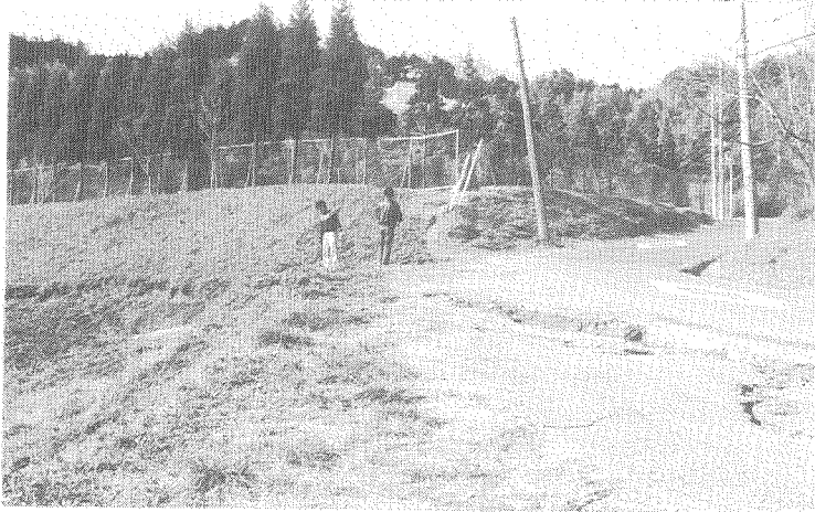
Photo. 14 Cracks along the edge line of school ground (reclaimed ground ) and cracks on the slope
