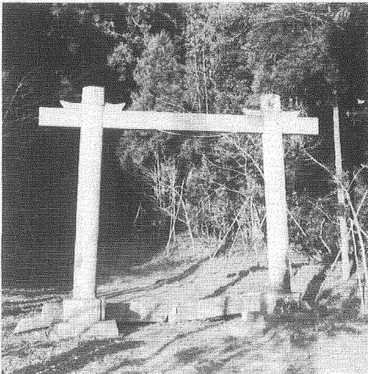
Photo. 19 Stone gate of Washizu Shrine (The upper part fell down on the ground)
