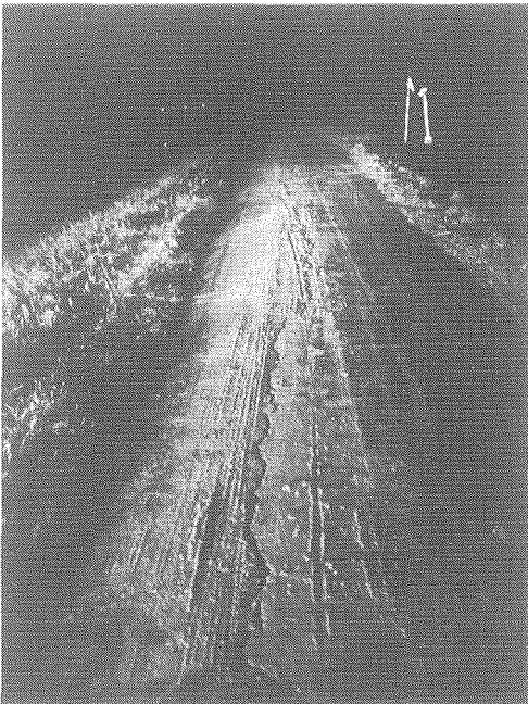
Photo. 12 Longitudinal crack on right side bank of the Tone River
